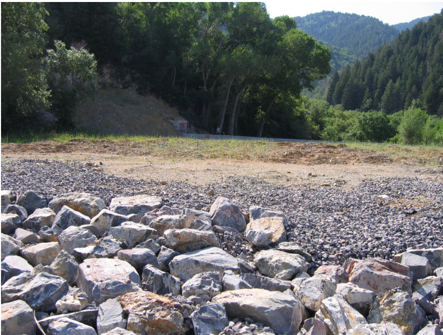
Figure No. 75: Pictured is the top of the Water Supply Tunnel Dump from near the top edge of the western embankment and newly reconstructed drainage channel. Surface revegetation was beginning to show better success.
