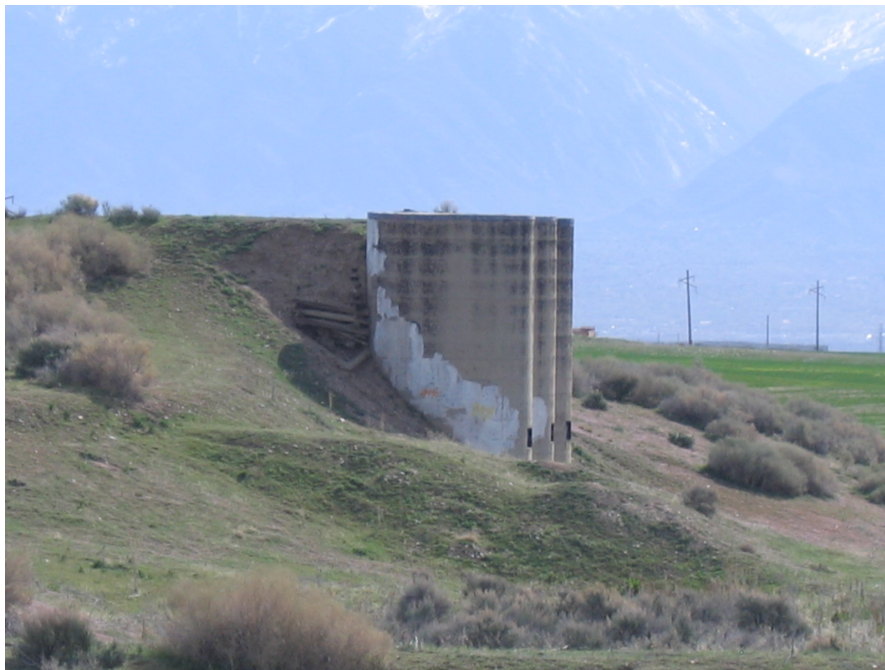
Figure No. 42: Pictured is the Midas Creek Silos area (Figure No. 46 is of the right side, or south side, of this area). Some removal action was performed in this area where once the Mascotte Ditch, Bastian Ditch and Midas Creek came together. The silos are still used for grain storage on a periodic basis and are visible from Rt. 111 (from where the photo was taken).
