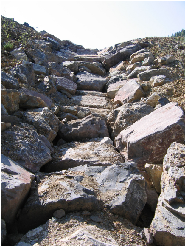
Figure No. 83: Pictured is a close-up of the drainage channel and its rip-rap near the top of the Water Supply Tunnel Dump. This channel was assessed to be stable for the limited water it potentially will receive draining from the top surface of the Water Supply Tunnel Dump.
