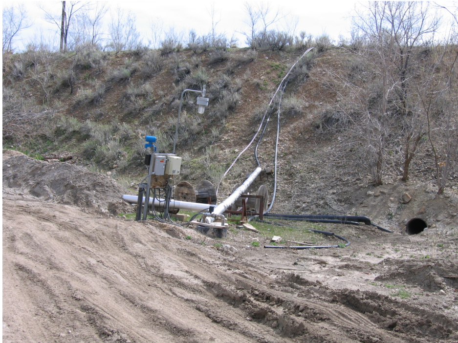
Figure No. 23: Pictured is the sump structure where tunnel produced along the length of the Mascotte Tunnel reports to be pumped to the water management facilities of Kennecott.
