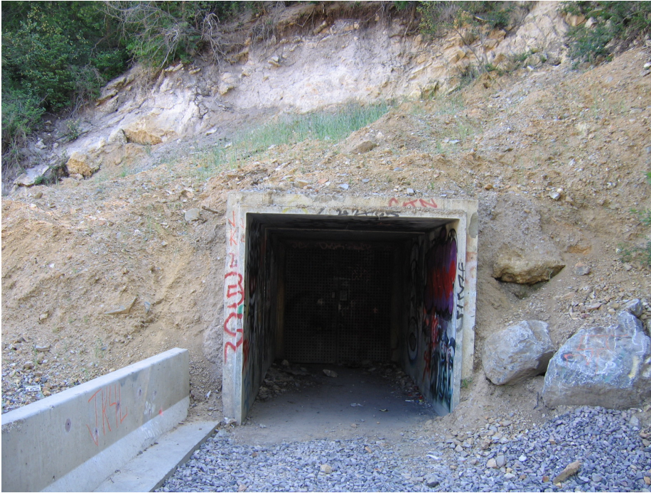
Figure No. 76: Pictured is the Water Supply Tunnel portal post reconstruction. A pipe inside the tunnel (since reconstruction) takes surface water produced from inside the tunnel's reaches down off the Dump and directs the flow into the local irrigation company's system (see Figure 41). A more solid steel door is inset from the concrete portal opening to allow access by the mine operators, but not the public.
