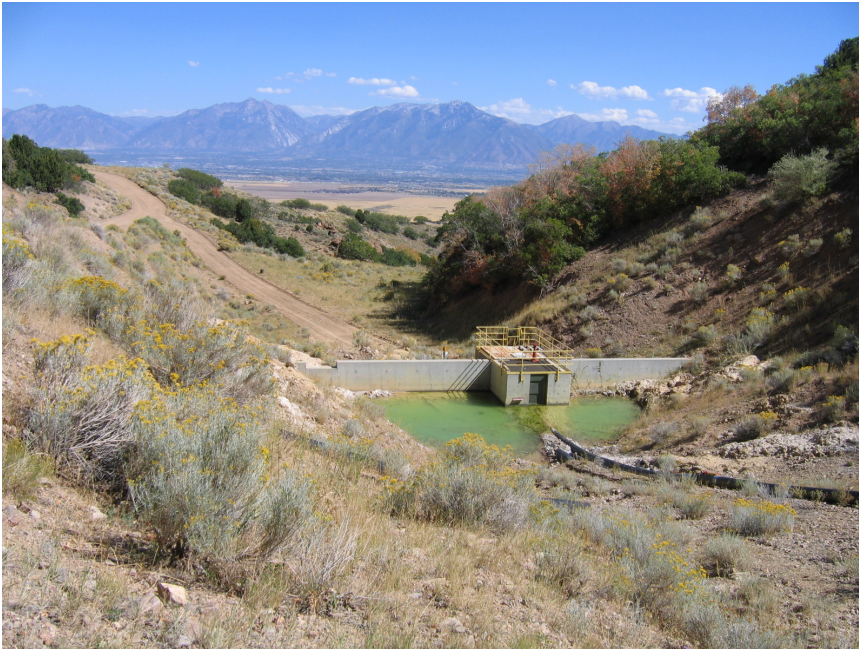
Figure No. 12: Pictured is the Yosemite drainage cut-off wall located approximately 100 yards down gradient of the sediment traps near the base of the waste rock dump.
