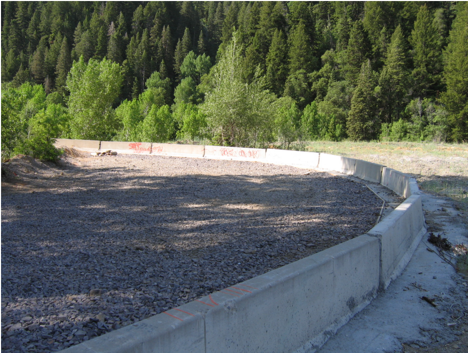
Figure No. 77: Pictured is the series of Jersey Barriers keyed into a concrete base from the tunnel portal to the eastern slope of the Water Supply Tunnel Dump. As of 2007 these barriers are used to keep the public from driving onto the \frac{3}{4} of the Water Supply Tunnel Dump's top surface. This barrier was installed to facilitate the revegetation effort.
