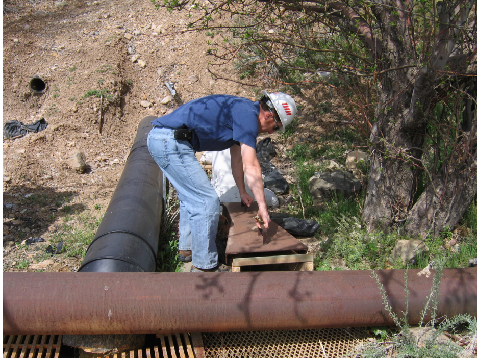
Figure No. 29: Mr. Kelly Payne is checking the historic flume that used to transport Bingham Tunnel water to the water management drop box; now the black HDPE pipe does.
