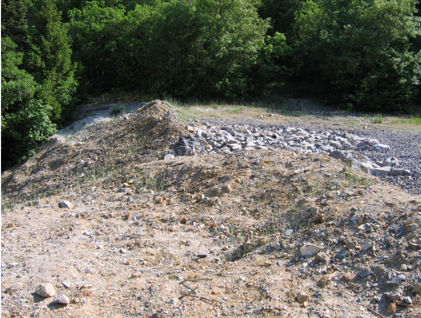
Figure No. 82: Pictured is the top section of the reconstructed drainage channel and capture area along the top edge of the western slope of the Water Supply Tunnel Dump. Top to bottom this drainage channel is significantly armored with rip-rap to protect it against undercutting. Note the water directional berm as part of the water control structures on top of the Dump.
