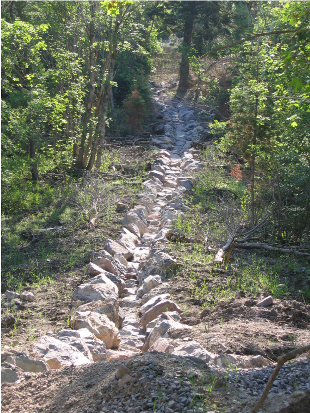
Figure No. 84: Pictured is the reconstructed drainage channel taken from the base of the channel near the water tank and irrigation system. Water from this channel is delivered to Middle Canyon Creek. Vegetative success near and along the base of the Water Supply Tunnel Dump is the best along the western and eastern slopes of the Dump.
