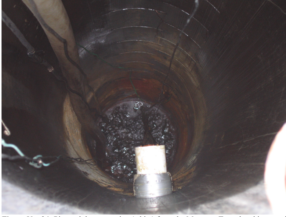
Figure No. 24: Pictured the water pipe (white) from the Mascotte Tunnel and its associated sump, water quality is okay for the copper extraction process.
