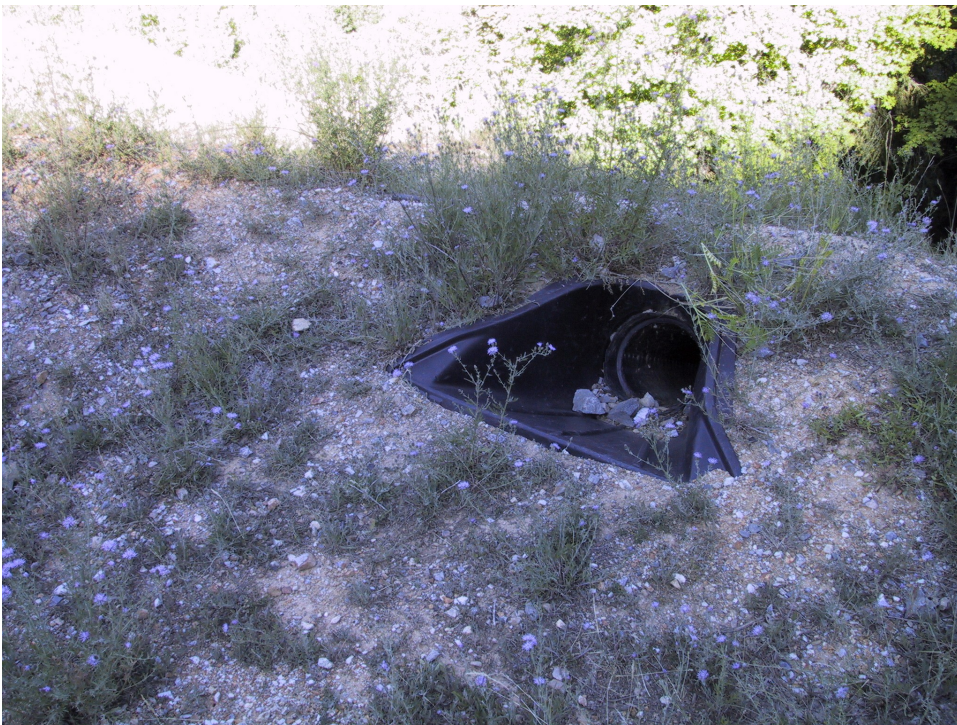
Figure No. 73: Pictured is the drain/catch basin for surface water flowing from the Water Supply Tunnel across the top of the Dump surface. In 2006 this catch basin was seen to be undercut by excessive water pushed out from the tunnel during its reconstruction.
