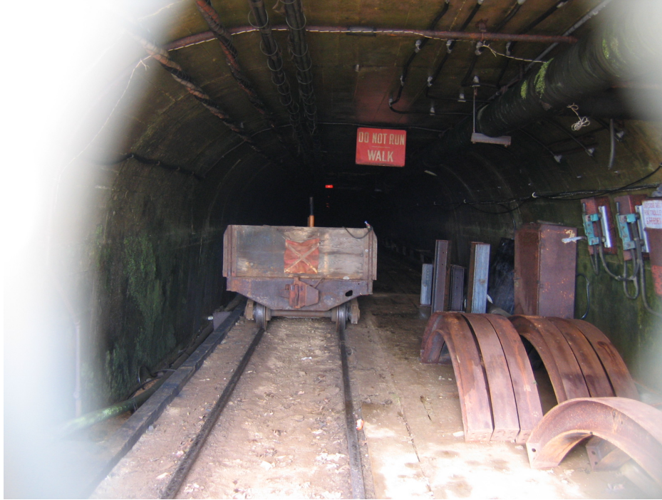
Figure No. 27: Pictured is the Bingham Tunnel just inside from the portal. Immediately to the right of the arched cribbing material is a tunnel that leads to the basement of the USSRM administration building. The tunnel is currently undergoing repair to replace some slipping sections of the cribbing. The waste rock produced from drilling this tunnel and the Mascotte Tunnel was the source of the waste rock found at Lark.
