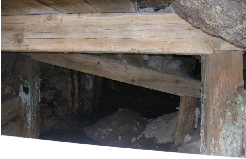
Figure No. 22: Pictured is the Mascotte Tunnel working just inside from the portal. The cribbing along this tunnel is wooden and in sections is in disrepair but the tunnel still produces water. The Mascotte Tunnel is down gradient from the Lower Keystone Drainage and cutoff wall.
