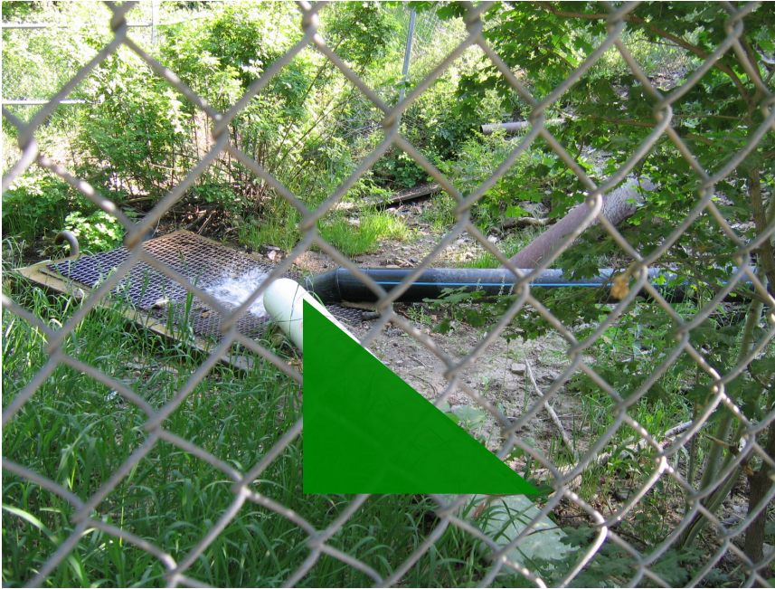
Figure No. 86: Pictured is the black HDPE pipe directing water from the Water Supply Tunnel straight into the local irrigation company's collection point off of Middle Canyon Creek. The green triangle is inserted in the frame to cover some publicly inappropriate graffiti on the white PVC pipe.
